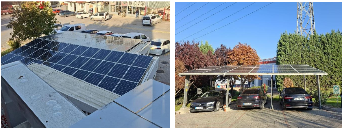
Solar panel located at the back yard and the car park of OSTIM Foundation
